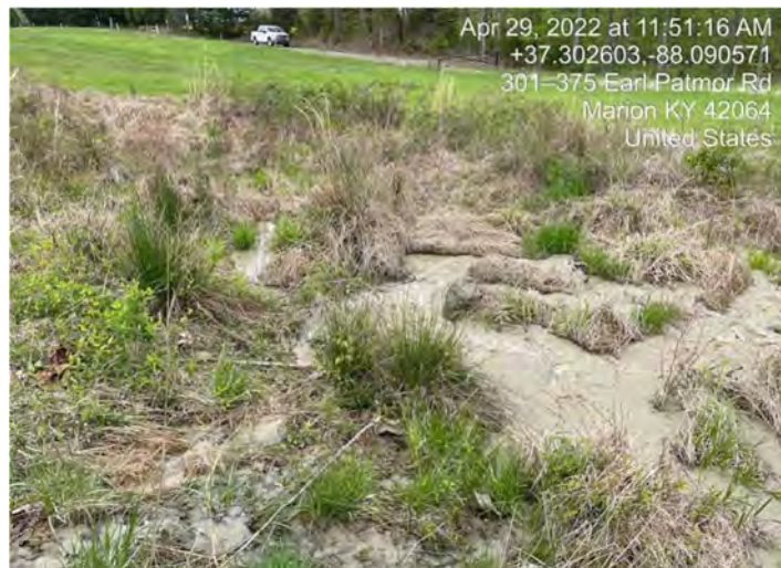
Figure 3. Turbid Boils and Seepage near Toe of Dam
