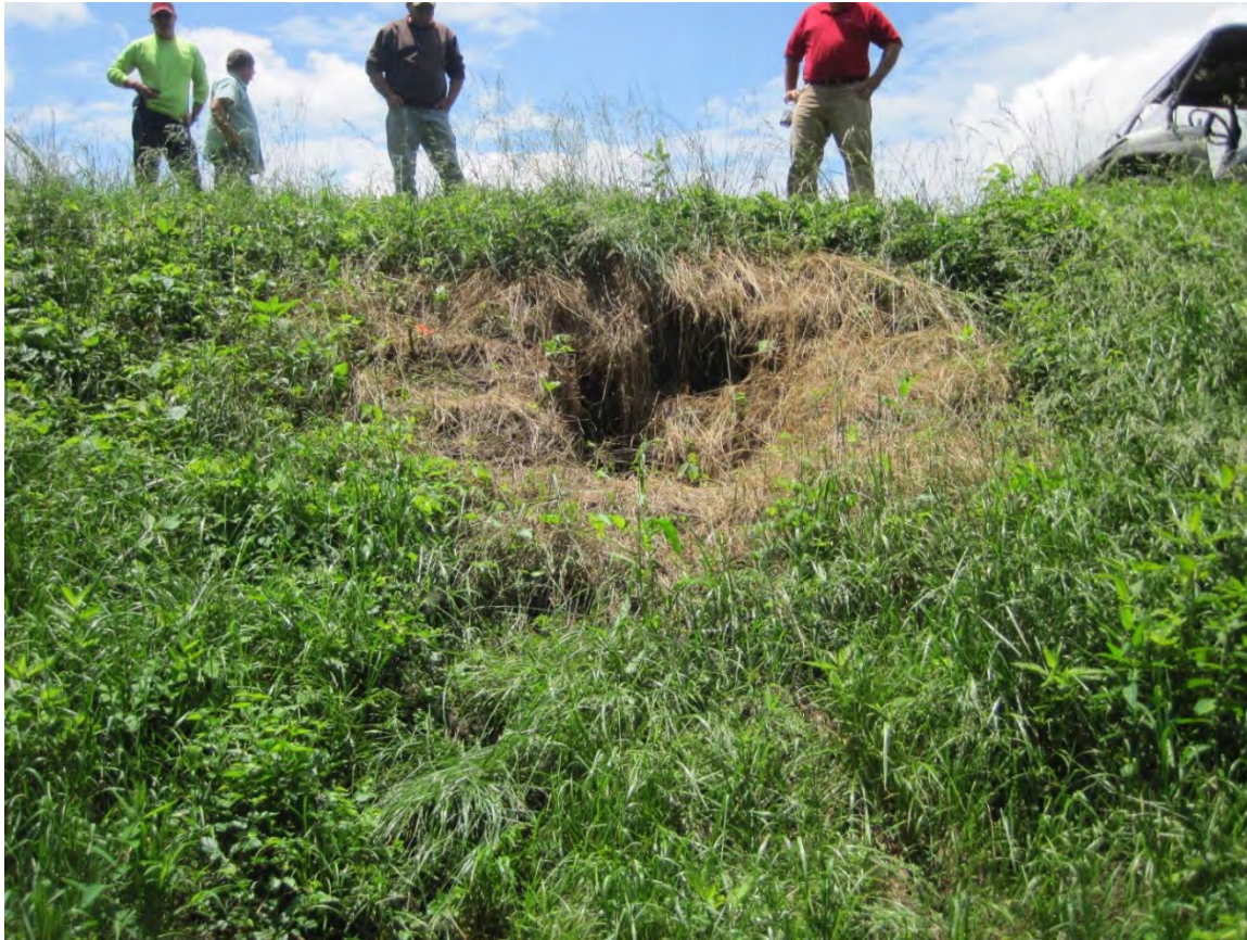
Figure 40. Riverside Slope Subsidence
