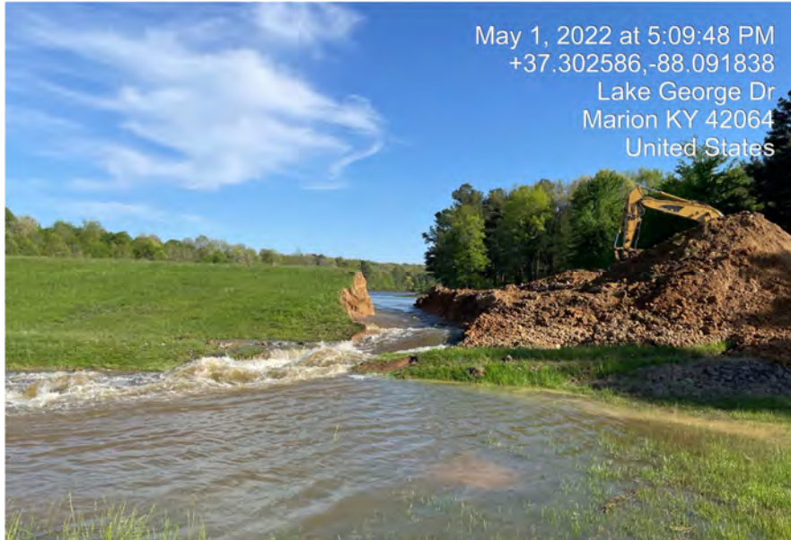
Figure 6. Breach Channel at Left Abutment
