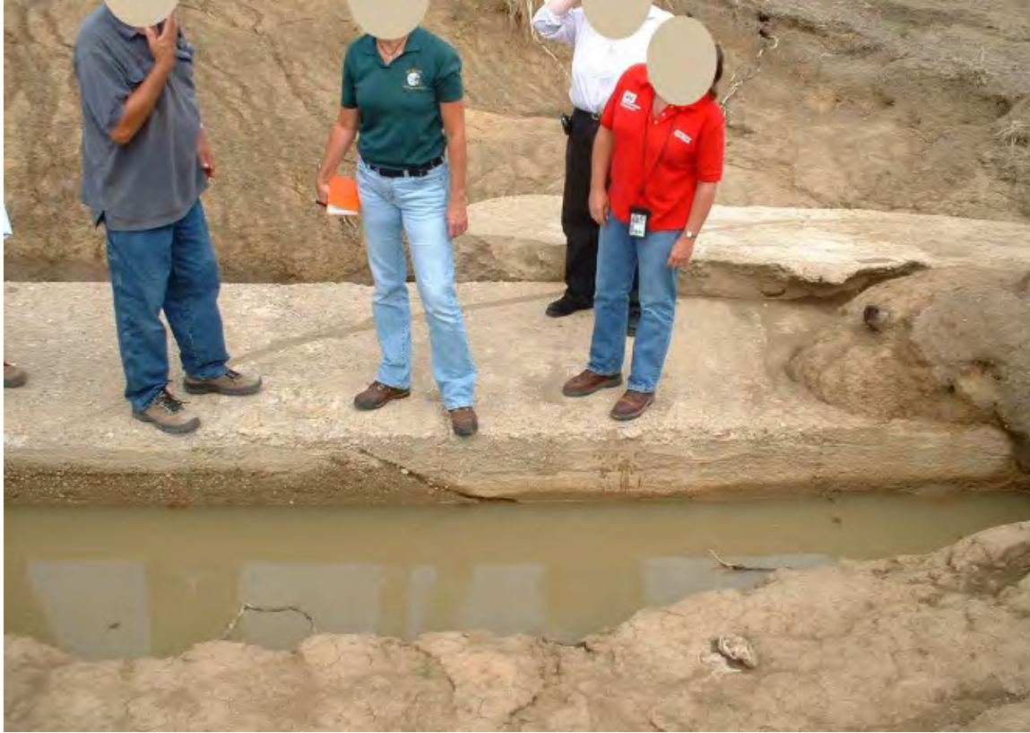
Figure 6. McGinnis Levee Failure with Crack in Concrete Culvert
