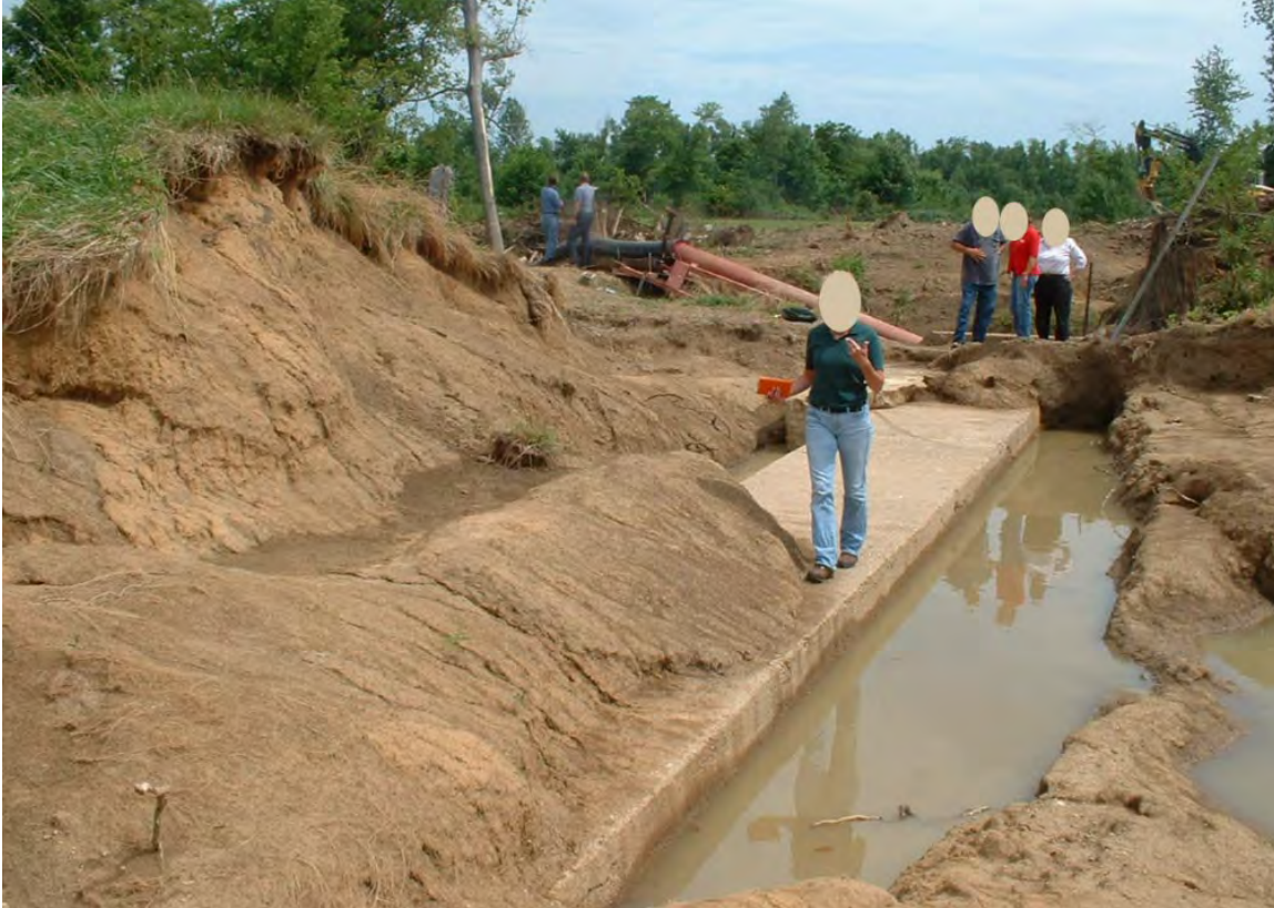
Figure 5. McGinnis Levee Failure looking toward White River
