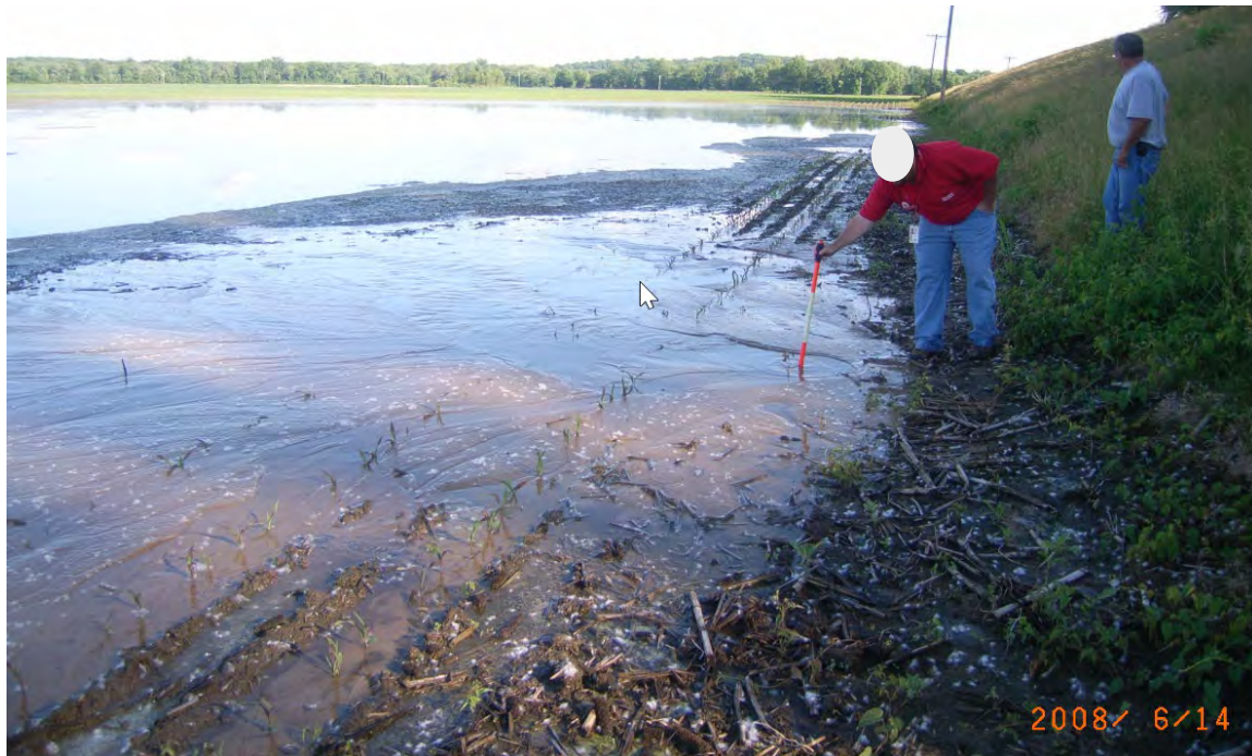
Figure 19. Large Boil During Flood Event at Landside Toe
