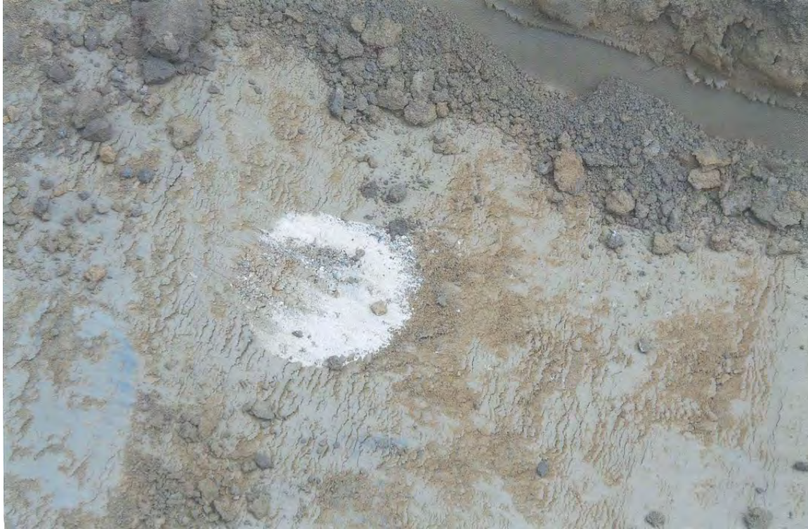
Figure 42. Boil Excavation Following Flood
