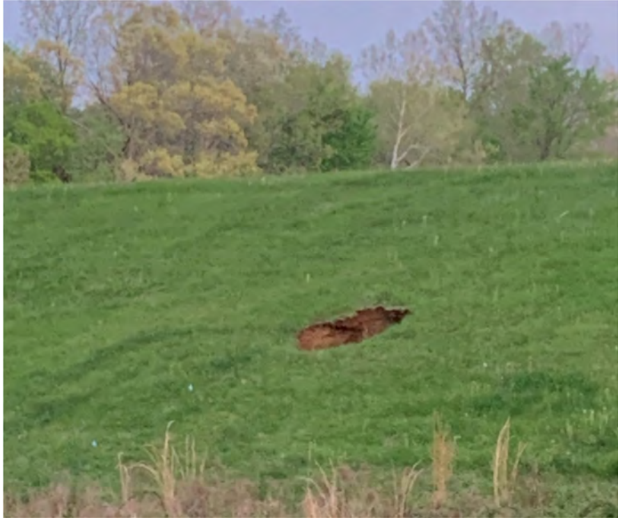
Figure 4. Sinkhole Immediately after Initial Development
