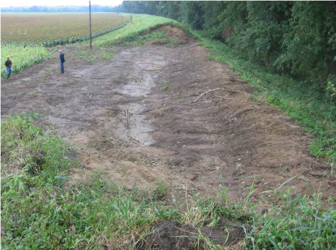
Figure 13. Russell Allison Breach Post-Inspection Photo
