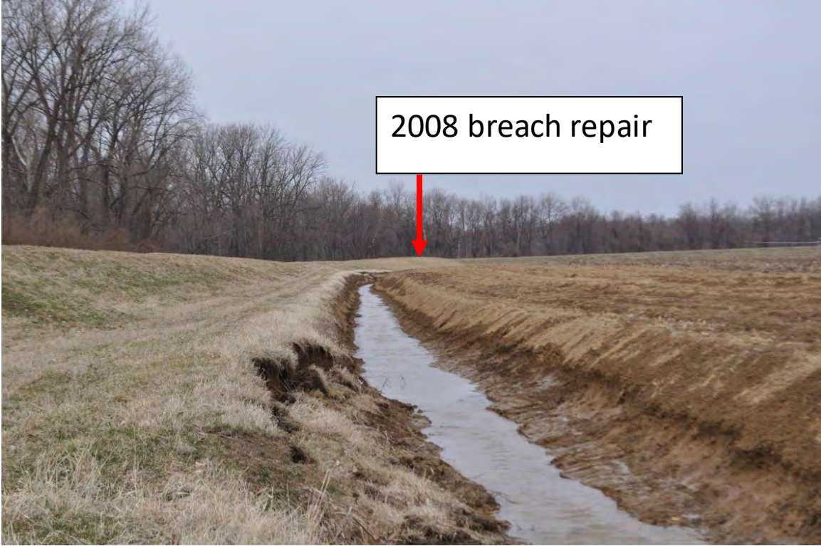
Figure 27. Levee Unit 8 with Sloughing in Landside Ditch
