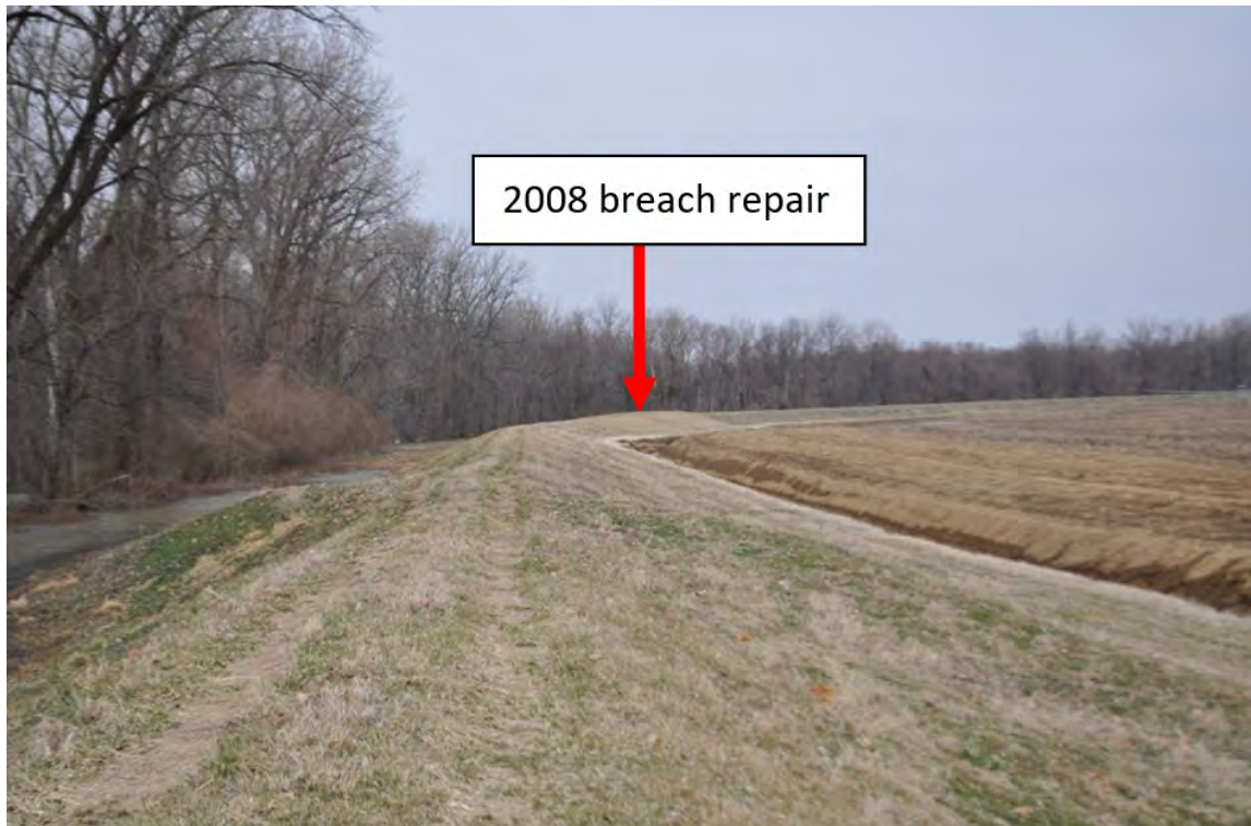
Figure 29. Breach location of Levee Unit 8 in Foreground and 2008 Repair in Background
