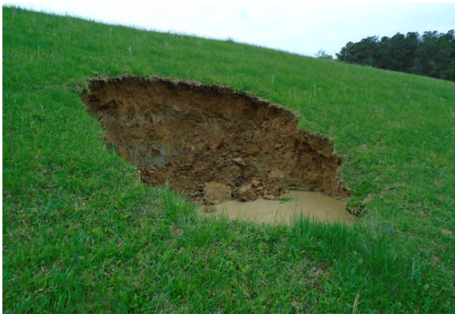
Figure 5. Enlarged Sinkhole after 24 Hours
