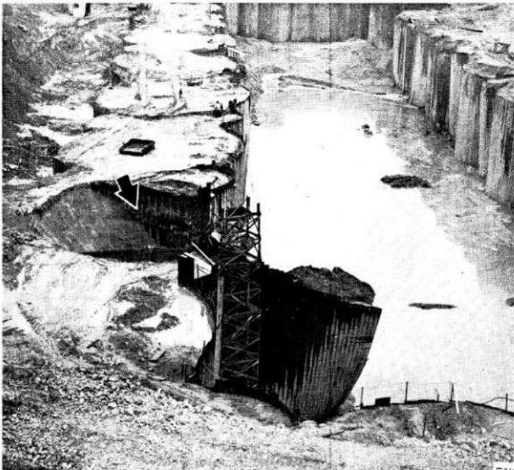
FAILURE AFTERMATH (arrow). Flooding and sand dumping stabilized cells.
