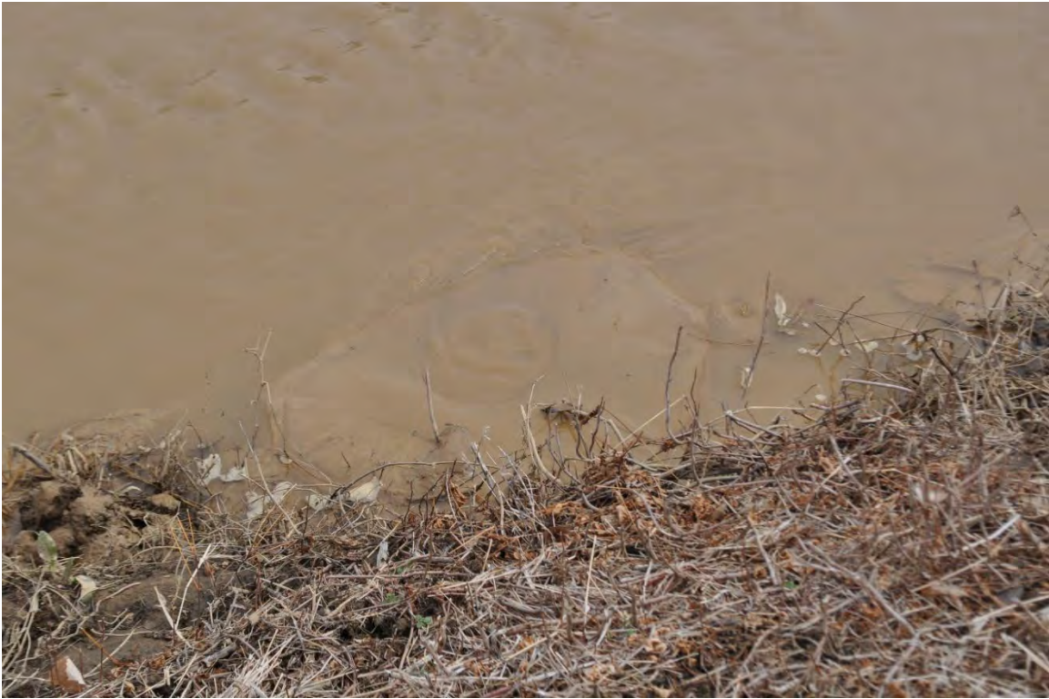
Figure 28. Boiling and Material Discharge within Landside Ditch
