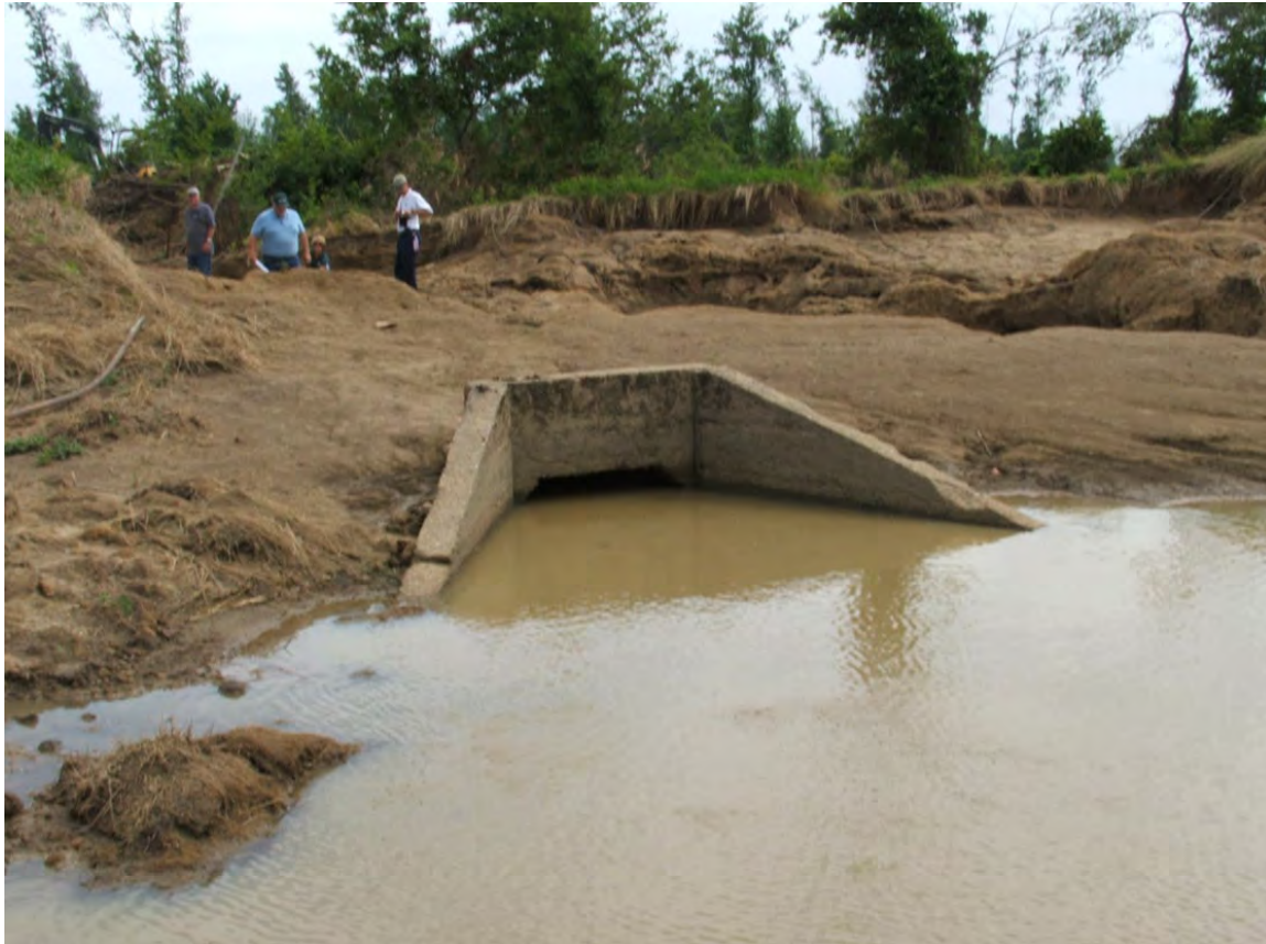
Figure 11. McGinnis Levee Failure Landside Headwall
