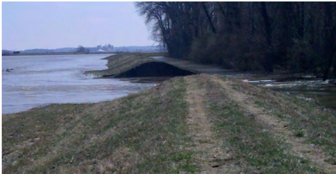
Figure 26. Levee Unit 8 Breach March 4th 2008 Looking Downstream
