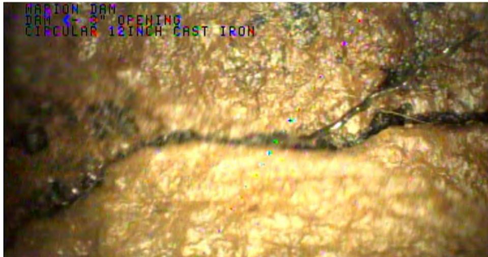
Figure 9. Crack in 12-inch CIP Interior Sidewall
