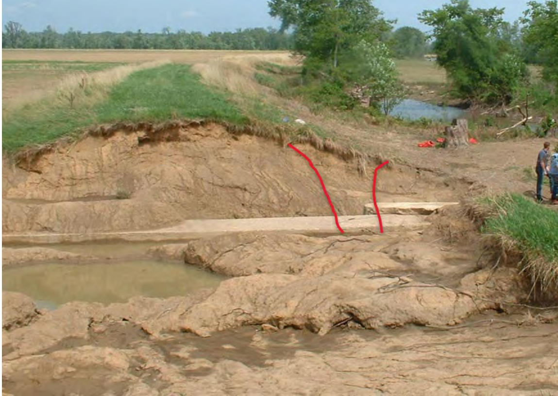
Figure 7. McGinnis Levee Failure and theorized Slope over Flaw in Culvert
