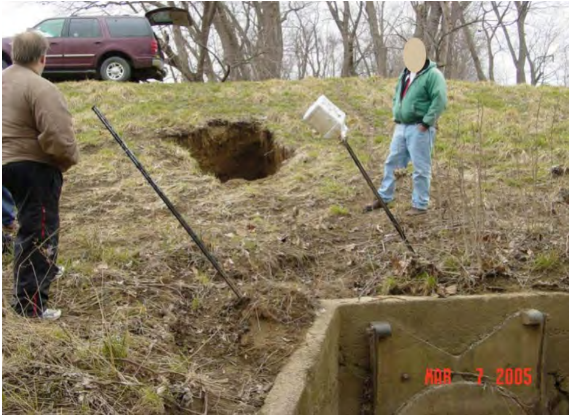
Figure 8. McGinnis 2005 Levee Collapse at Different Culvert Location
