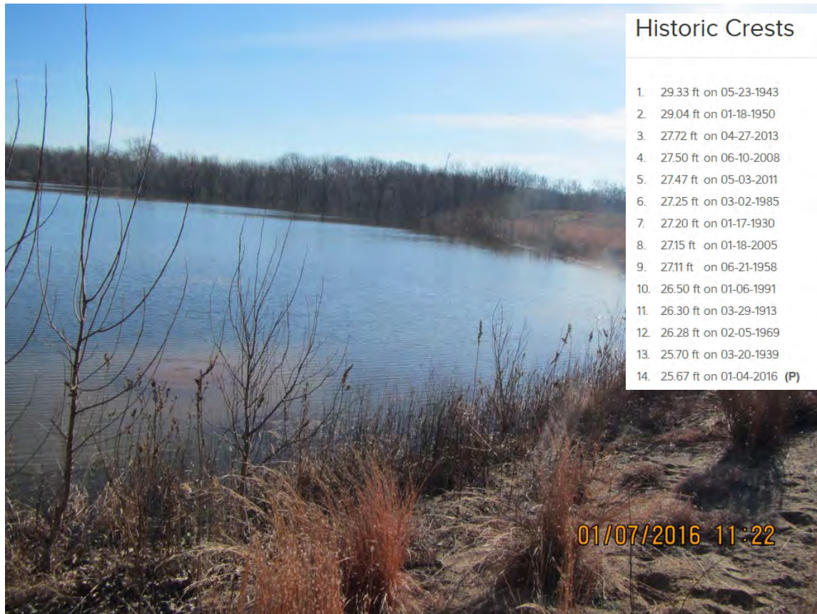
Figure 24. Photo of Toe of Niblack Sand Berm and Large Boil from 2016 Flood
