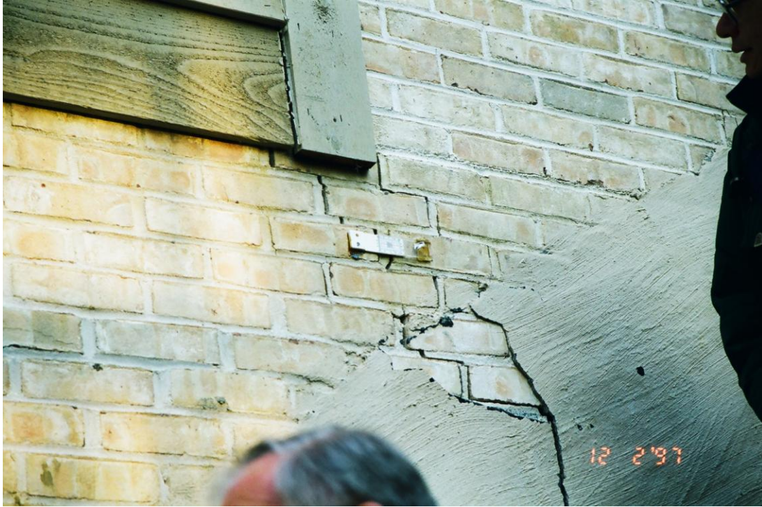
Fig. 7. Cracks in west wall.
