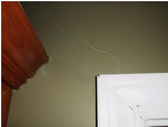
Fig. 5. View of jagged crack above doorway.
