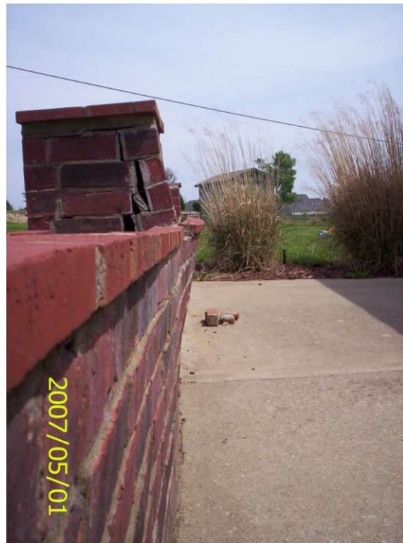
Fig. 24. Post-blast photo of brick planter. Roadcut being widened is between the wall and the house in the background.
