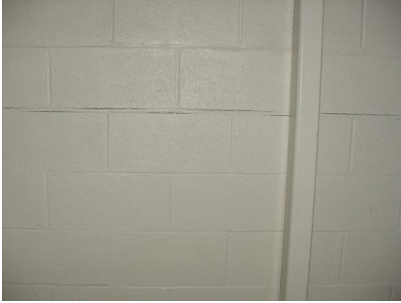
Fig. 13. Horizontal cracking behind steel tube column in garage.
