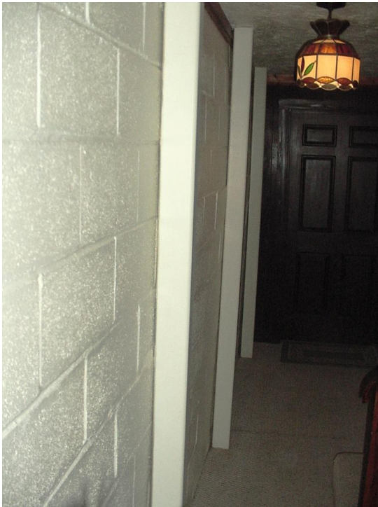
Fig. 15. View of inward buckling of wall restrained by steel columns.
