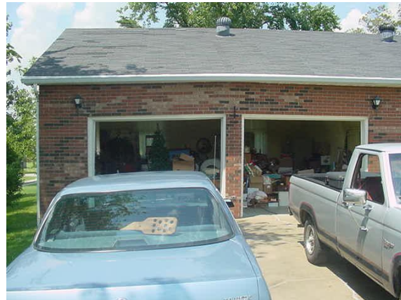
Fig. 42. Settlement of slab-on-grade garage corner caused by seasonal moisture extraction from mature tree off left side of photo.
