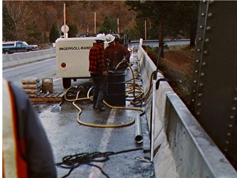
Fig. 15. After placing the cable, grout was tremied into the hole below the footing and into the steel pipe between the top of footing and top of pier
