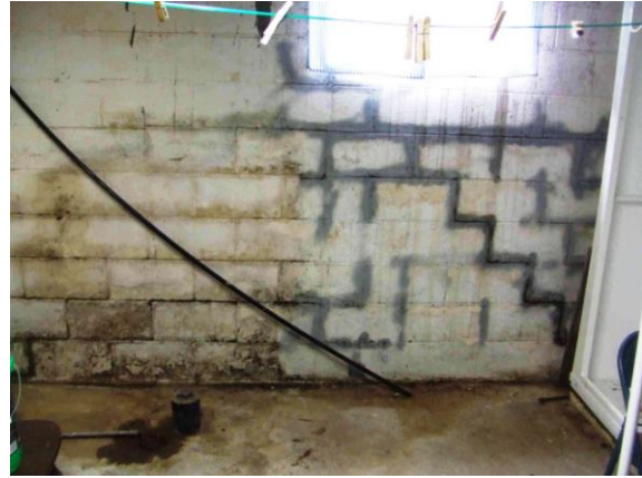
Fig. 34. Water damage visible to west basement CMU wall. This wall has bowed inwards under active earth and hydrostatic pressures.
