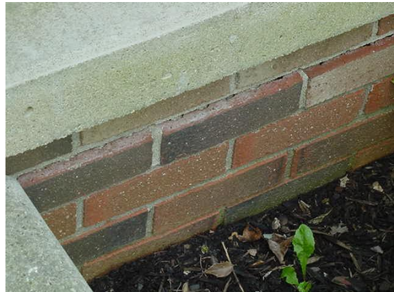
Fig. 40. Short front porch wall has stayed in place while front porch slab is dragged to the rear along with the first floor.
