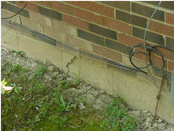
Fig. 39. Depression in ground surface resulting from inward buckling of front basement wall.
