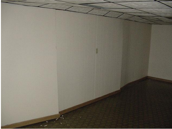
Fig. 35. View of buckled basement walls and drop ceiling.
