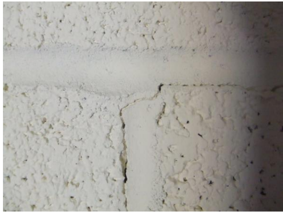
Fig. 12. View of year-old paint filling crack space.
