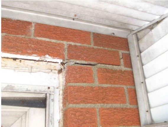
Fig. 33. Horizontal cracking caused by expansion of rusting steel lintel at top of door frame.
