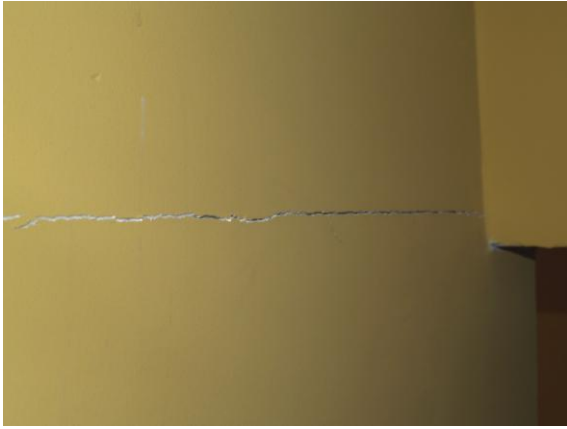
Fig. 25. Jagged horizontal crack in interior stairwell.
