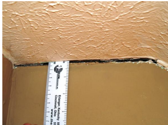
Fig. 28. Jagged crack at ceiling of second-floor dormer, showing lateral offsets.
