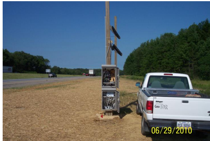
Fig. 10. The head ends of the eight spliced coaxial cables were connected to the data acquisition system (DAS)
