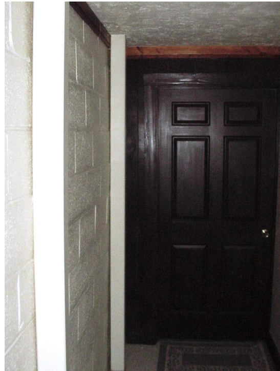
Fig. 16. Another view of inward wall buckling restrained by steel columns.
