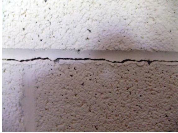
Fig. 10. View of 1.6-mm (1/16-inch) horizontal offset in crack.
