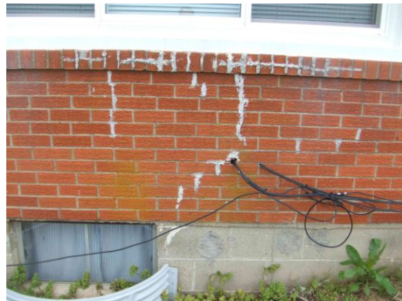
Fig. 32. Previously-caulked damage beneath picture window.
