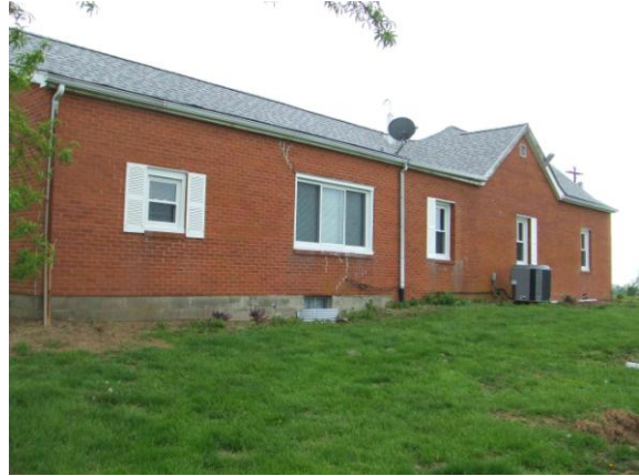
Fig. 30. West wall of house. Heaviest damage to brick façade occurs over partial basement (see window well).
