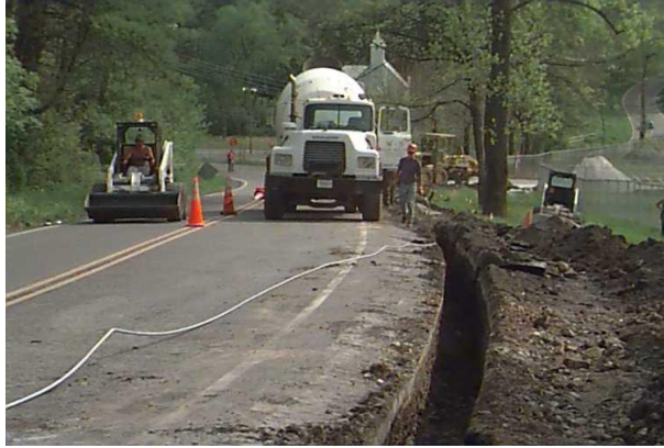
Fig. 2. Installing cable in a trench along SR 91; cables were also installed in angled holes drilled below the road from the berm (see Fig. 3)
