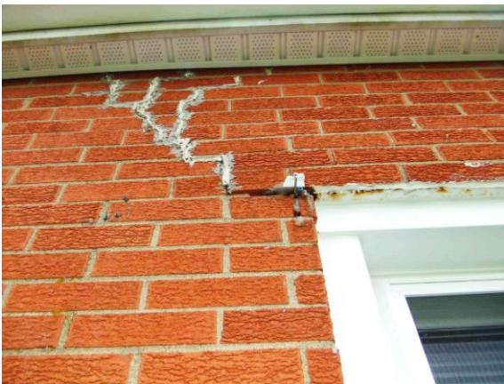
Fig. 31. Previously-caulked damage over upper left corner of picture window. Subsequent movement has squeezed caulk out of cracks.
