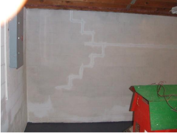
Fig. 3. Previous repairs visible on basement walls.
