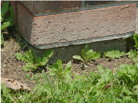
Fig. 37. Horizontal offset in brick on rear wall caused by thrusting of first floor to the rear.
