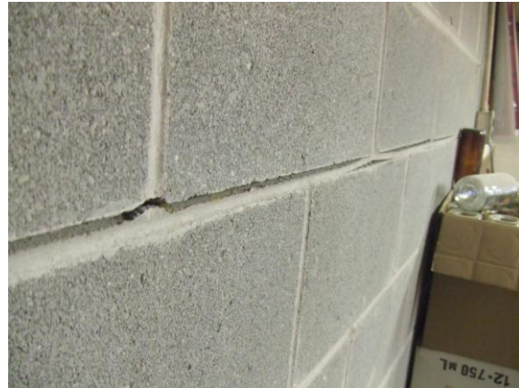
Fig. 2. View of inward bowing of replaced portion of basement wall.
