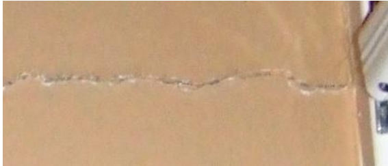
Fig. 17. View of jagged crack at upper left window corner.
