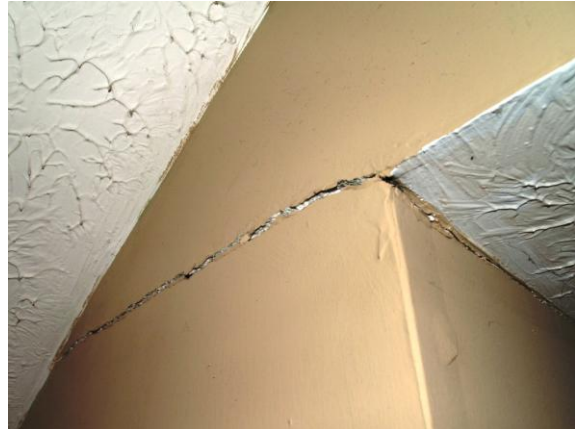
Fig. 26. Jagged crack near ceiling between stairwell and entry to second-floor bedroom.
