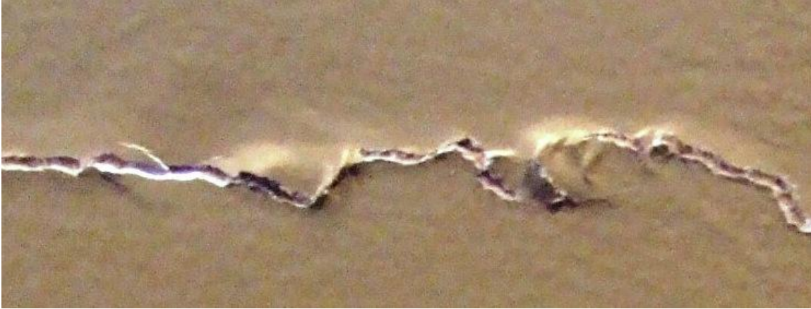
Fig. 21. Closeup of crack shown in Fig. 20, showing horizontal offset and crushing of drywall caused by shear.
