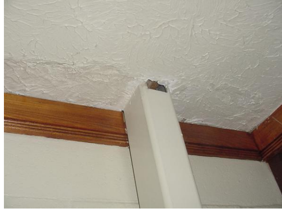
Fig. 14. Evidence that column was installed after basement was finished.
