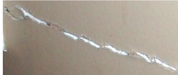
Fig. 18. Closeup of jagged crack shown in Fig. 19.
