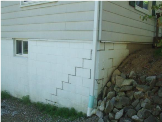
Fig. 1. Non-replaced corner of basement walls, showing previous tuckpointing.
