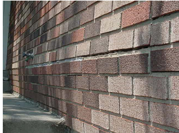
Fig. 38. Buckling of brick façade on rear wall caused by thrusting of first floor to the rear.
