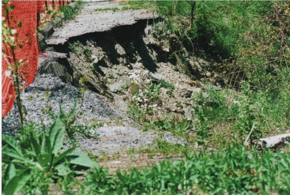
Fig. 1. North end of the ground movement on May 22, 1997
