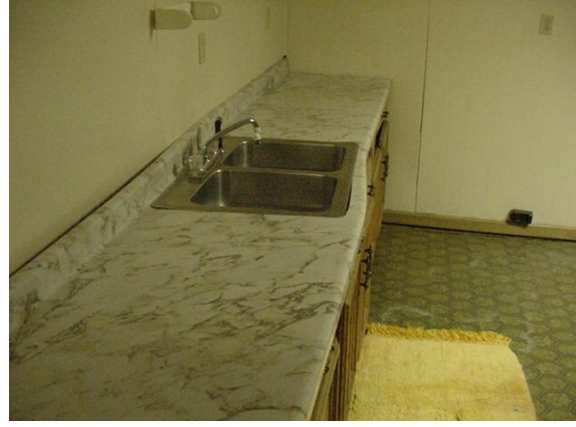
Fig. 36. Buckled basement wall caused buckling of kitchen countertop.
