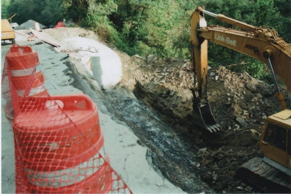
Fig. 11. Block of concrete placed at the north end to avoid rock excavation
