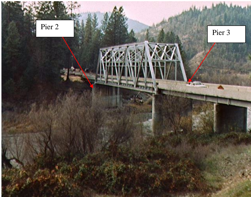
Fig. 14. Bridge over Klamath River; scour pocket developed under Pier 2 in the background; cables was installed through the foundation of Pier 3 in foreground.
