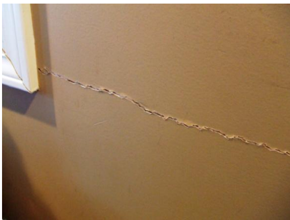
Fig. 19. View of jagged crack at lower right window corner.
