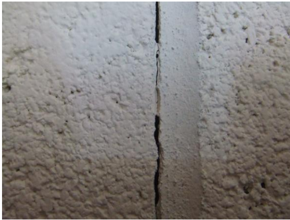
Fig. 11. View of year-old paint spanning sides of crack.
