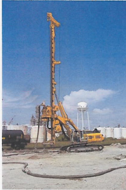
FIGURE 13 Texas City CMC installation site.
