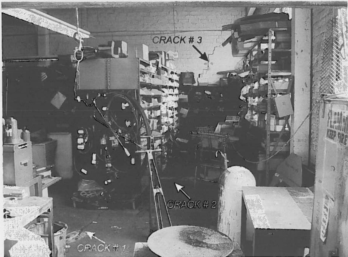
Figure 5: Locations Of Interior Cracks Monitored During The Press I Construction
