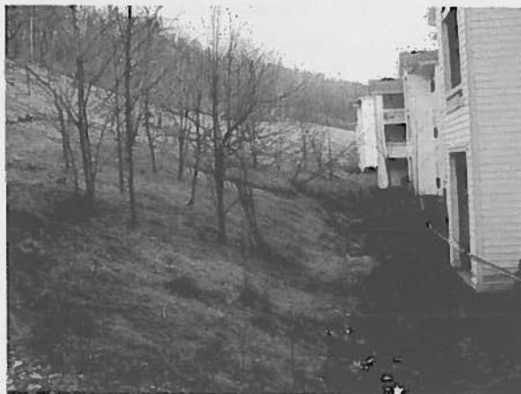
Figure 2. Early warning signs, small bulges in the slope.
