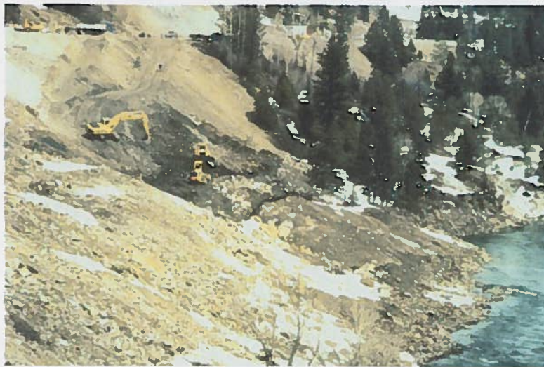
Figure 1. Blue Trail Landslide site, April 1997
