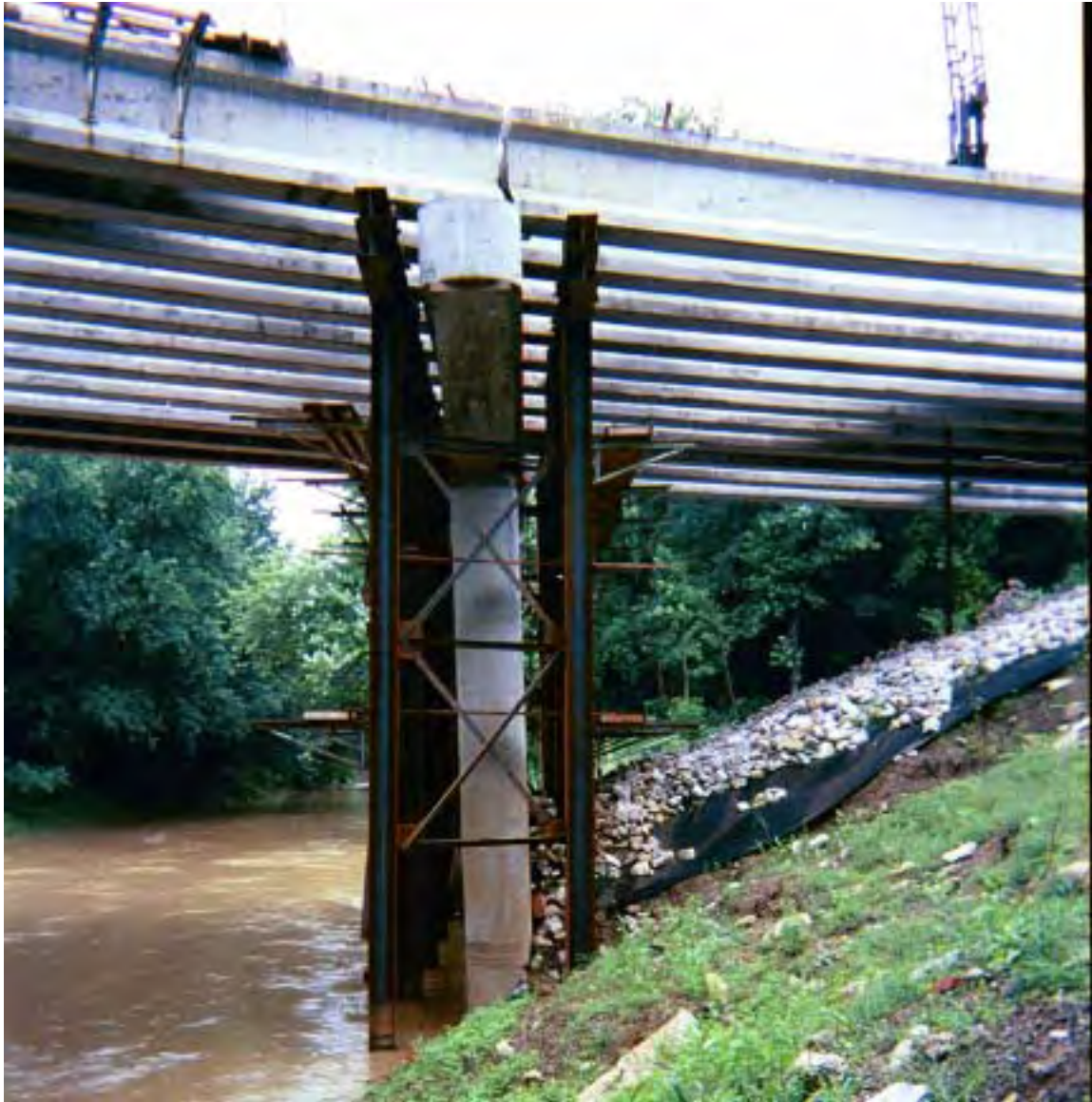
Photo. 1. Interior pier (No. 3), looking west (taken after temporary support of the pier was provided)
