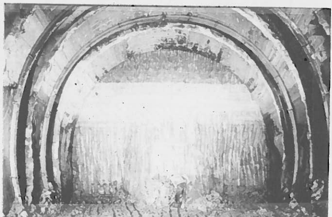
Figure 5. Concrete, shot into the pre-cut slots, creates overlapping concrete shells of conical shape. When required, steel ribs can be added for extra strength as shown.
