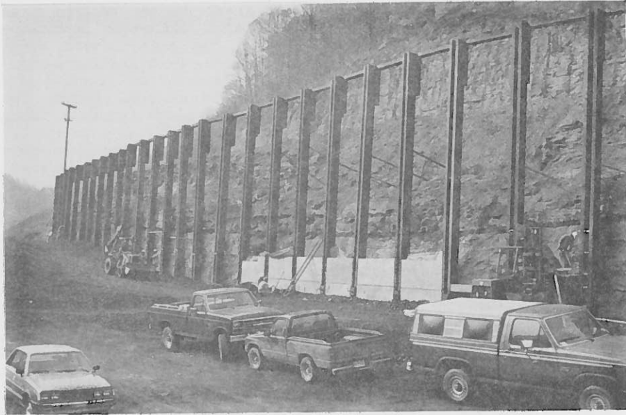
Figure 8. Photograph of erected double beam sections and initial precast concrete panel placement.
