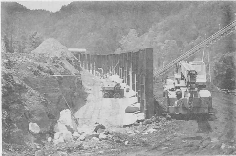
Figure 9. Photograph of backfilling operations behind wall and coal pile access in front of wall.
