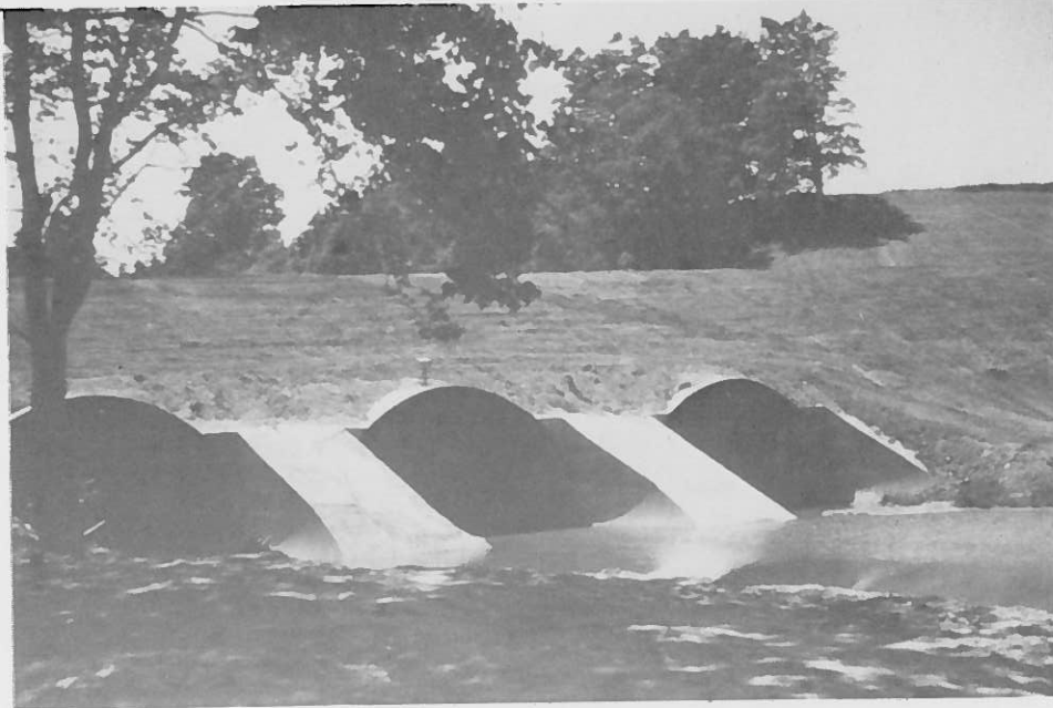
Figure 1. Three Armco Long-Span Horizontal Ellipses with 27-ft Rise, 37-ft Span, and 29-ft Height of Cover
