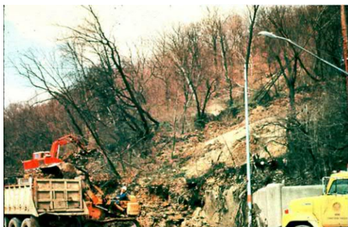
1975 Landslide (Photograph Courtesy of City of Cincinnati)
