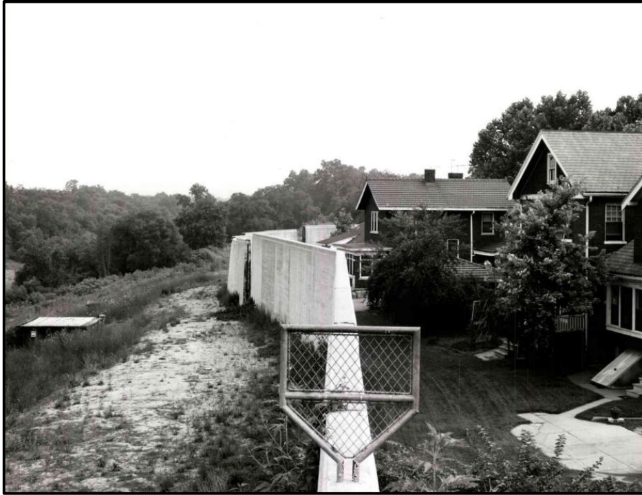
Figure 11: Looking south toward displaced monoliths (Drainage Pit No. 4 to the left)
