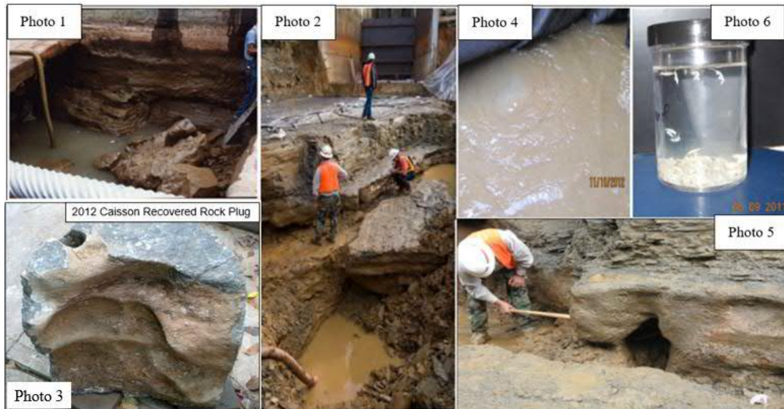
Fig. 6. Photo 1 – 1984 Repair, Photo 2 – 2007 Repair, Photo 3 – 2012 Caisson Excavation in BCLS, Photo 4 – 2012 Artesian Flow, Photo 5 – 2007 BCLS Karst, Typical, Photo 6 – Water Sample from Weep Hole with Freshwater Isopods.
