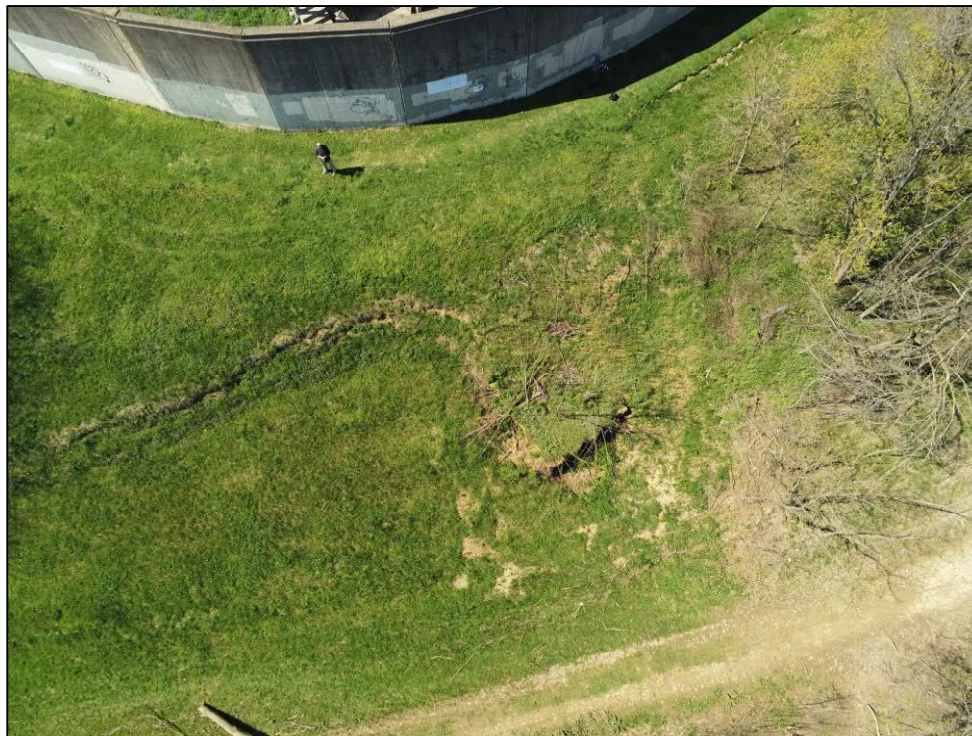
Figure 17: Slide scarp in January 2021 viewed from UAV over the riverside slope
