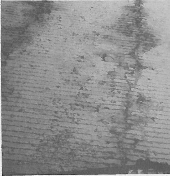
Longitudinal Cracks (Medium to high severity)
