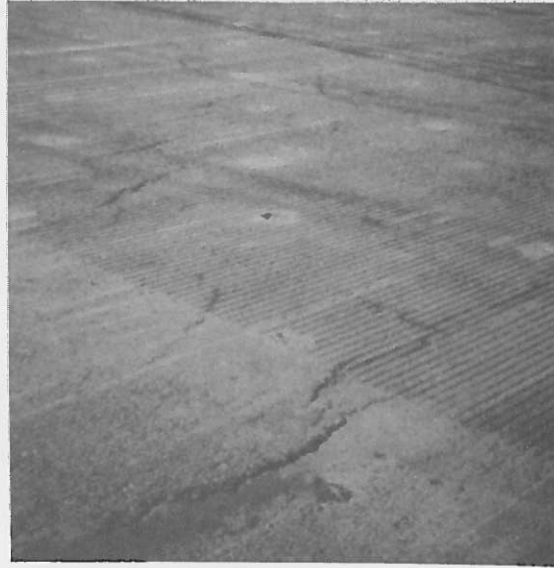
Block Cracks (Low severity)
