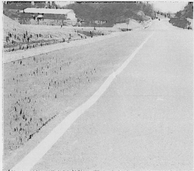
Figure 29. View of pavement and crack heave on Ky Route 11 near station 280+00
