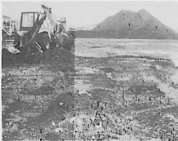
Figure 3. Photograph showing typical soil-cement pad failures
