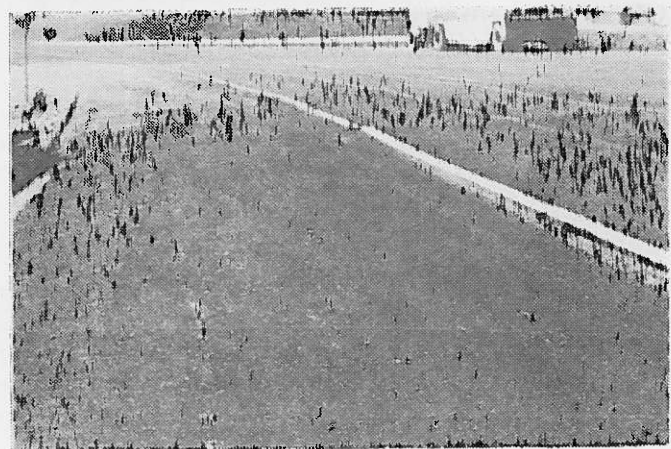
Figure 30. View of pavement humps on Ky Route 11 near station 560+00
