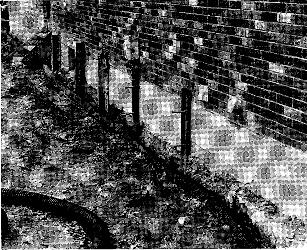
FIG. 5. Homeowner's Remedial Measures at Toe of Slide Area.
