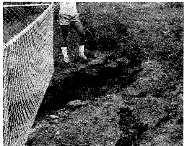
FIG. 11. Seep Near East End of Toe.
