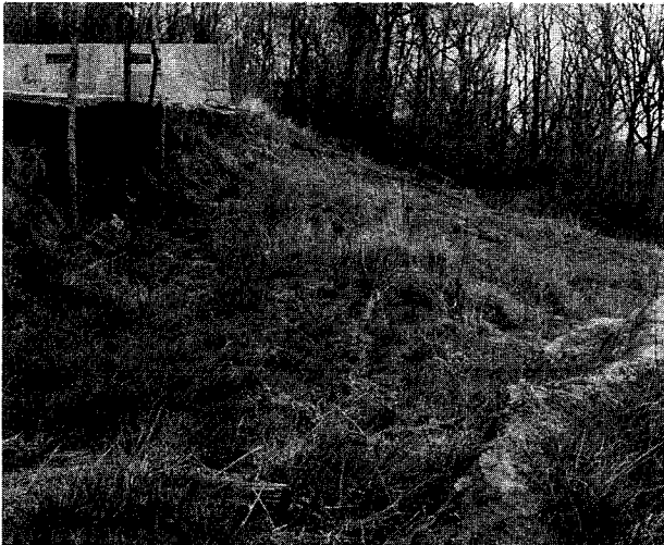
FIG. 3. Retreat of Scarp Under Demolished House.
