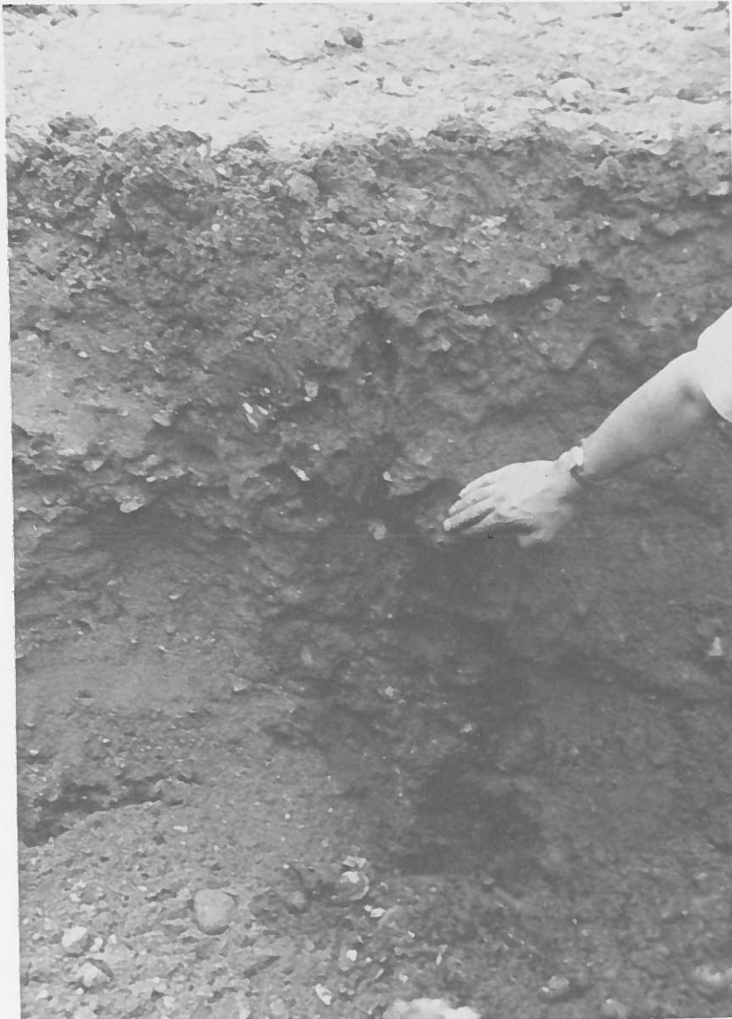
FIGURE 17 LOOSE SAND PIPE EXPOSED ON VERTICAL SURFACE
