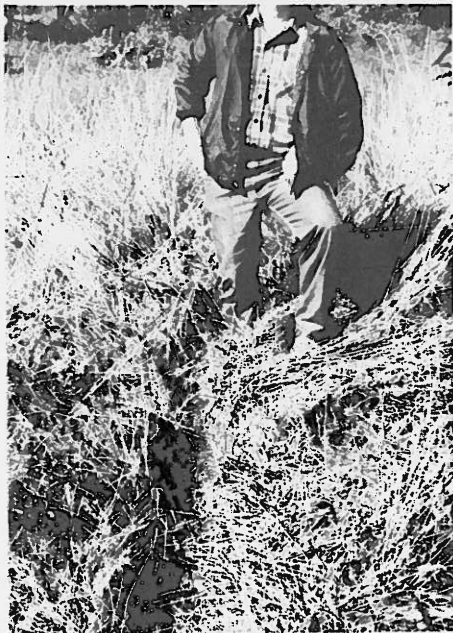
Figure 6. Crack (dark area in grass) in thin veneer of soil over rock along west rim of reservoir near Old Ben No. 26.
