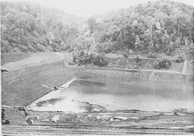
Figure 3. Slurry impoundment after Stage 1 upstream construction. Slurry line is relocated to discharge at embankment (Site 1).
