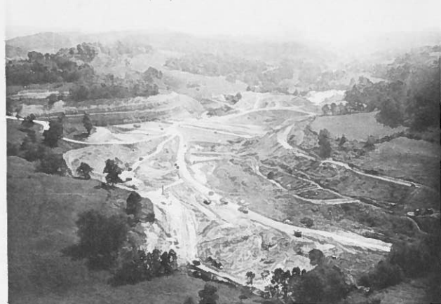
Figure 6. Borrow material being hauled to embankment. Note filter fabric between earth and rockfill zones of embankment in background (Site II).
